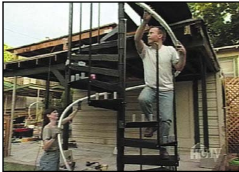
Nancy and Curtis are pictured above installing the handrail on their metal spiral stair kit.
